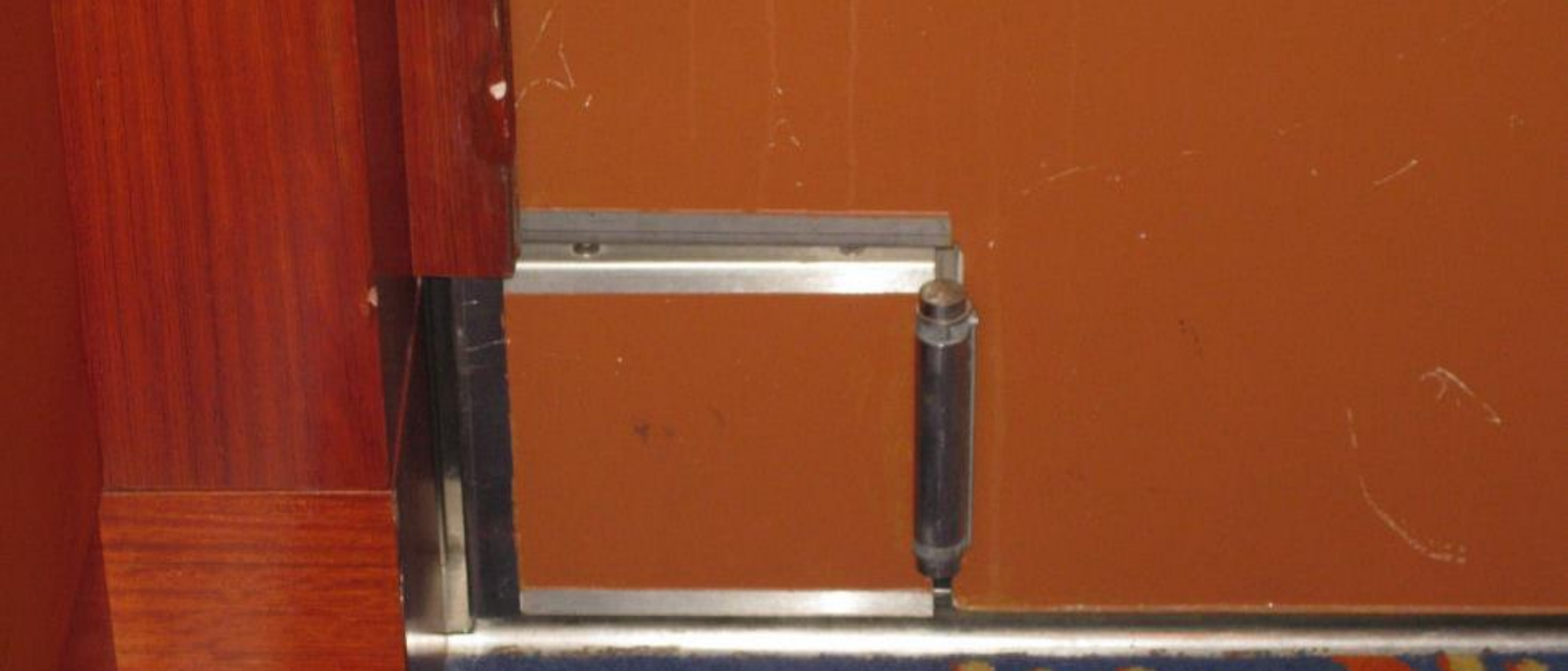
Hose Port in Fire Screen Door
